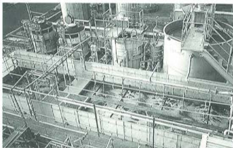
Henkel Hokusui Corporation: the efficiency of the biological stage of the sewage treatment plant was increased by more than one third.
